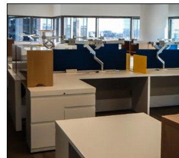
The work stations are coming together in the new 6th floor space.
